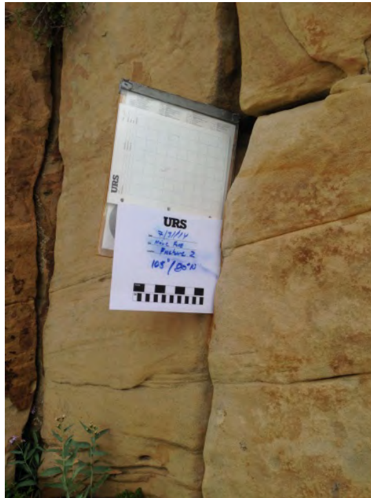
Photo 2. Fracture observed within mine portal area.
